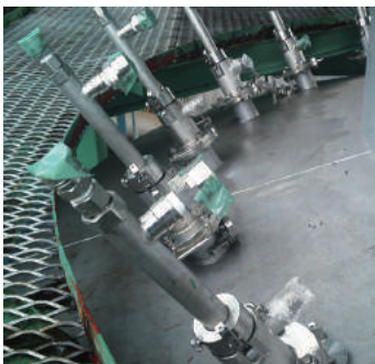
Nozzle installation locations in a cooling tower
