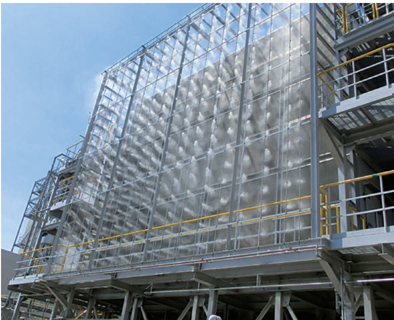
Semi-Dry Fog® inlet air cooling system (Photo courtesy of Shikoku Electric Power Company, Inc.)
